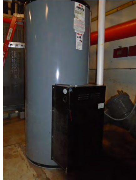
Fig. P-5 – Domestic hot water booster heater and storage tank
