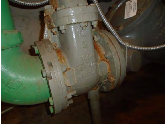
Fig. F-1 – Fire Entry main 8" shut-off valve
