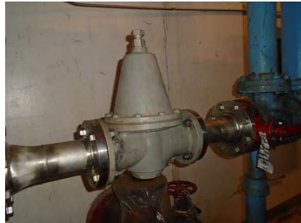
Fig. P-2 – Pressure Reducing Valve
