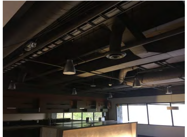
Fig. M-18 – Exposed mechanical infrastructure on fourth floor.
