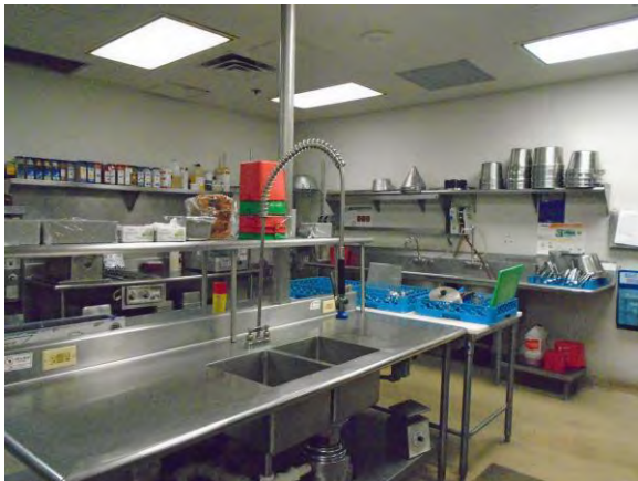
Fig. P-24 – Commercial kitchen sinks
