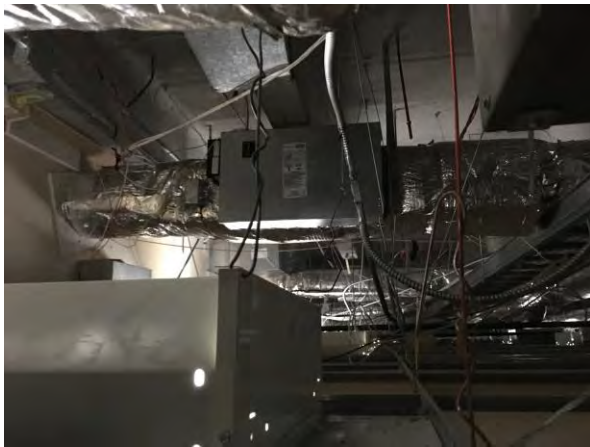
Fig. M-17 – Electric duct heater serving third floor west perimeter offices
