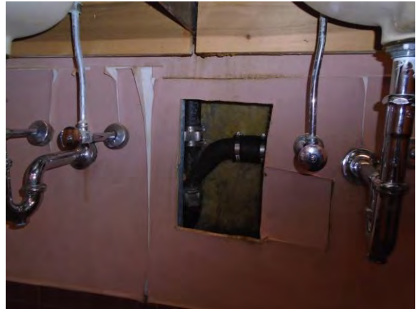
Fig. P-29 – Another example of access opening under lavatories
