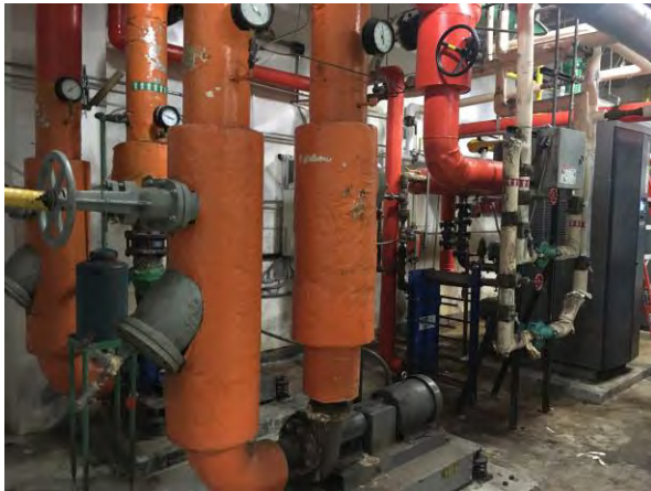
Fig. M-3 – Heating water secondary pumps shown in the lower left of photo and one of the boilers shown on the right side.
