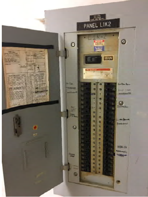
Photo #1: Kitchen Panel potentially requiring replacement.
