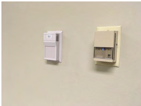
Fig. M-21 – Pneumatic thermostat alongside DDC zone sensor on wall of first floor conference room.
