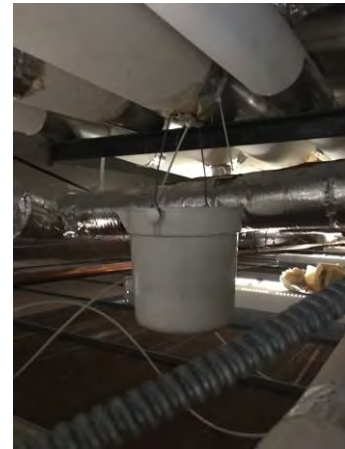
Fig. M-4 – Bucket found hanging below heating water pipe in the southwest corner of the second floor office space. This is evidence of leaking heating water piping.
