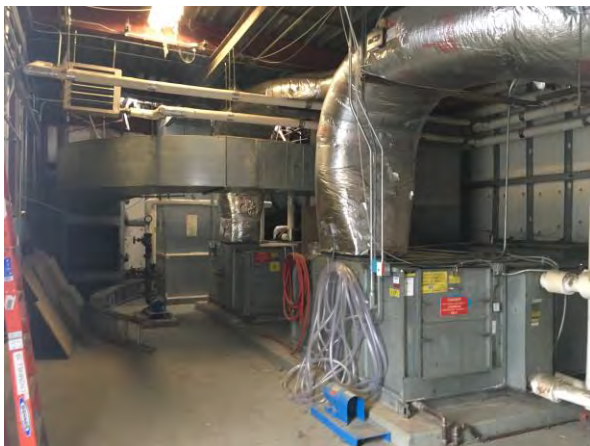
Fig. M-13 – Two (2) smaller penthouse air handling units serving perimeter induction units.
