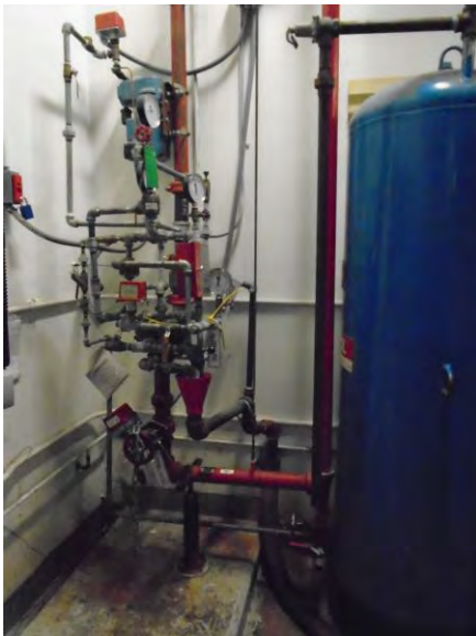
Fig. F-3 – Dry pipe valve assembly for dock sprinklers Located in mechanical room
