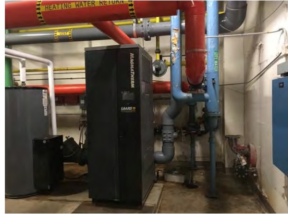
Fig. P-32 – Gas regulator (in back) in mechanical room
