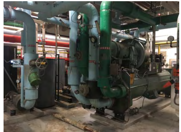
Fig. M-6 – Older Carrier chilled described as backup, not in operation.
