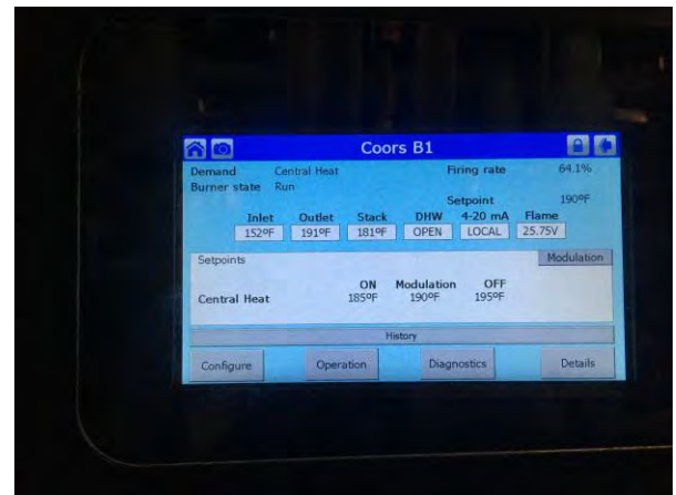
Fig. M-2 – Boiler operating conditions during second site visit.
