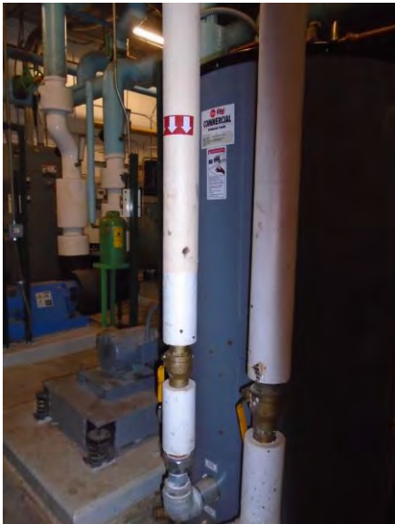
Fig. P-6 – Domestic hot water storage tank
