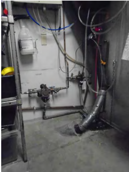
Fig. P-27 – Backflow preventors on 1 st floor
