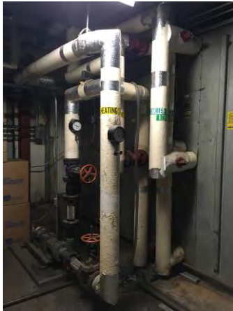
Fig. M-11 – Chilled water and heating water piping for penthouse air handling unit.
