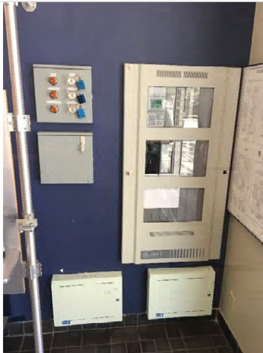
Photo #7: Fire Alarm Control Panel (Lobby)
