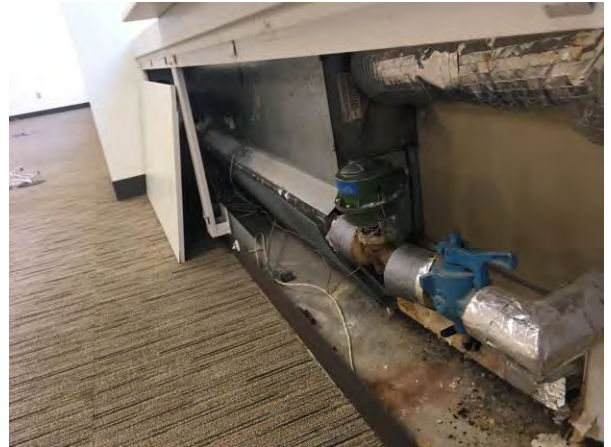
Fig. M-16 – Inside casing of typical perimeter induction unit.
