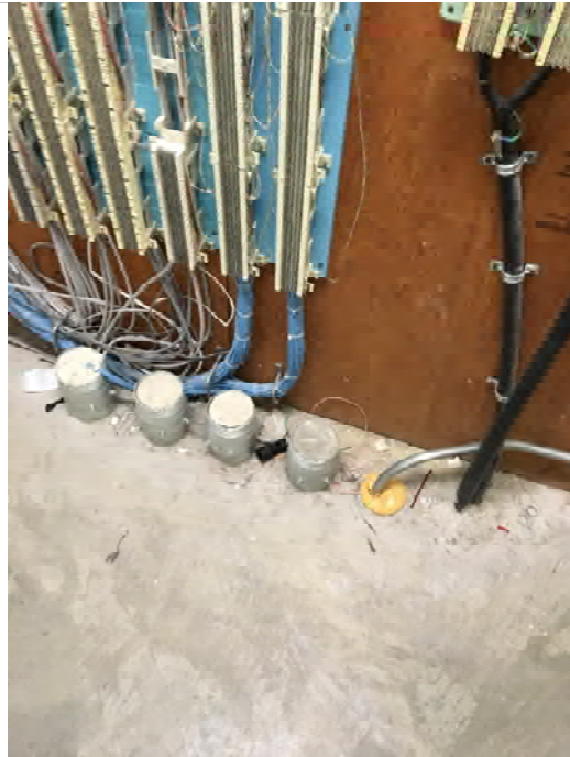
Photo #5: Existing IT Infrastructure
