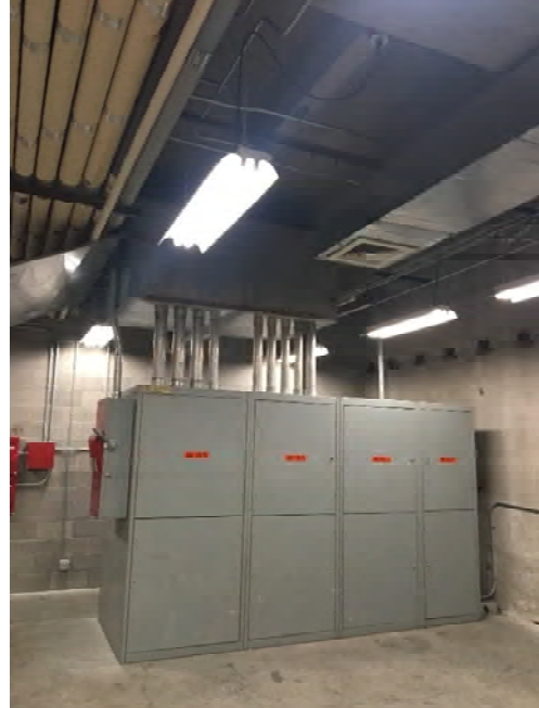
Photo #2: Main Electrical Room and MDC
