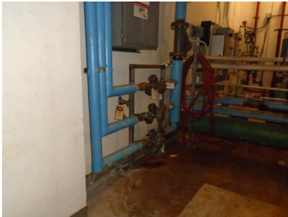
Fig. P-3 – (3) reduced pressure backflow preventors off main line
