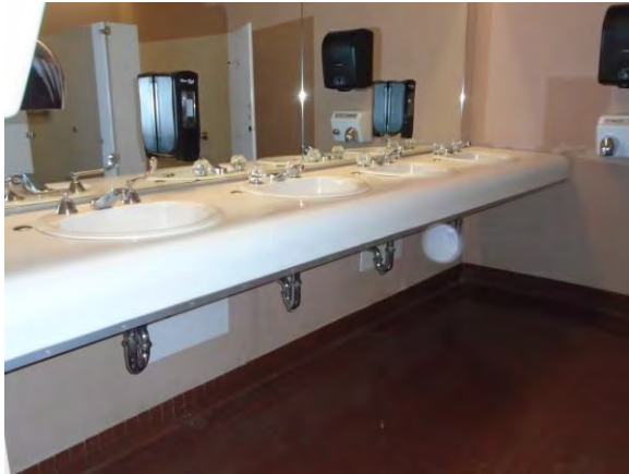
Fig. P-7 – Typical lavatories in restrooms
