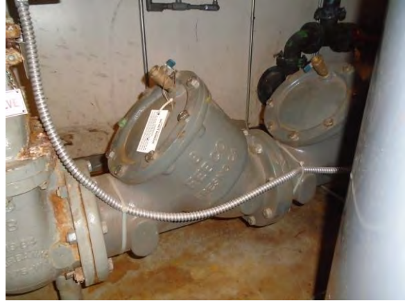
Fig. F-2 – 8" double check backflow preventor on fire line
