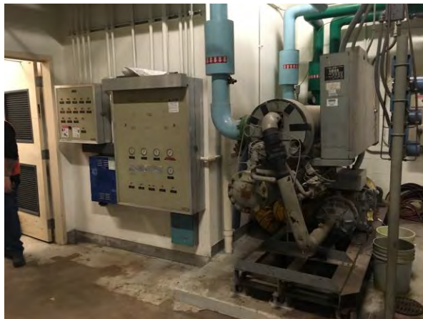
Fig. M-7 – Small abandoned chiller.
