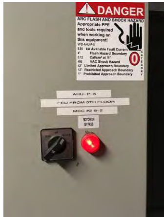
Fig. M-19 – Example of penthouse air handling unit VFD operating in bypass mode.
