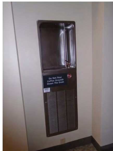
Fig. P-15 – Typical water cooler in office space
