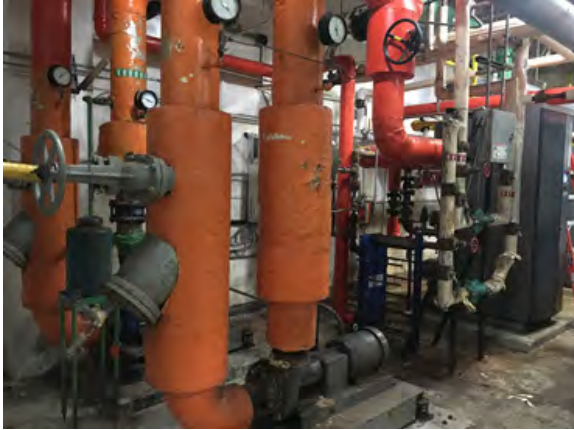
Fig. M-1 – Heating Water Secondary Pumps
