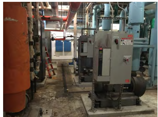
Fig. M-10 – Secondary chilled water pumps with VFDs.
