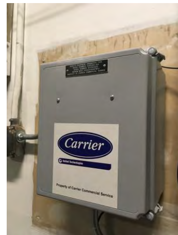
Fig. M-22 –Carrier control panel for newer chiller.
