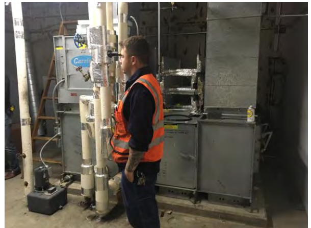
Fig. M-14 – Air handling unit serving recording studio.
