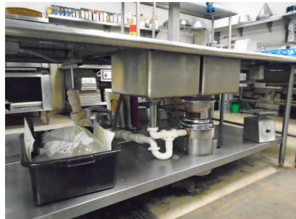
Fig. P-25 – Commercial garbage disposal
