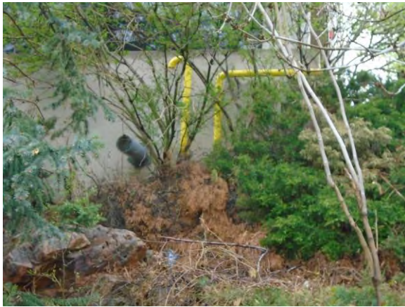
Fig. P-33 – Natural gas vent from regulator in mechanical room
