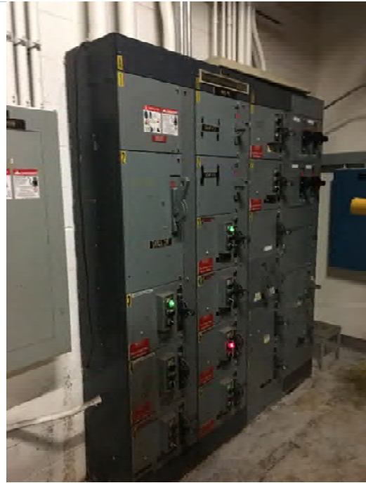
Photo #6: Motor Control Center #1 (MCC #1)
