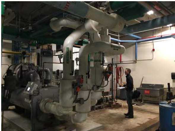
Fig. M-5 – 2011 Carrier chiller in operation.
