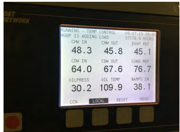
Fig. M-8 – Chiller operating conditions during second site visit.
