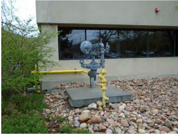
Fig. P-31 – Natural Gas entry
