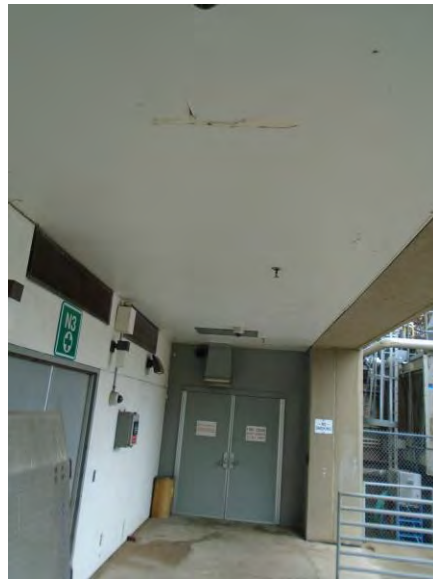
Fig. F-4 – Dry pipe sprinkler heads on dock
