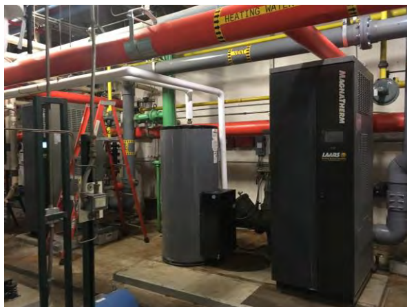
Fig. M-1 – Boilers shown on left and right of photo.
