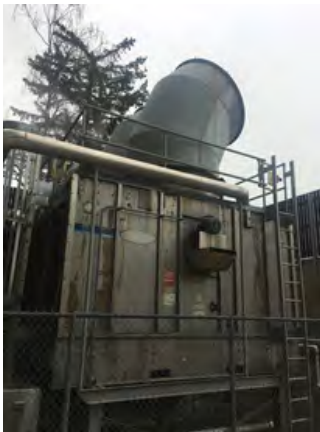
Fig. M-4 Two-cell Cooling Tower
