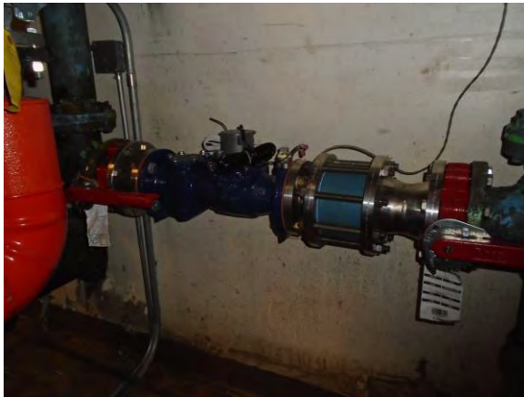
Fig. P-1 – 3" water meter at water entry
