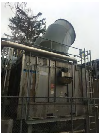
Fig. M-9 – Two-cell cooling tower located on the east side of the building.
