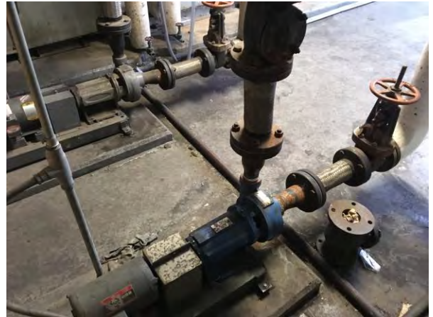
Fig. M-12 – Two heating water coil circulation pumps for two large penthouse air handling units.
