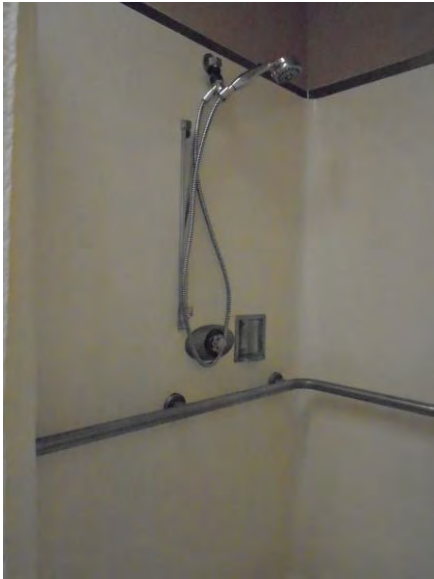
Fig. P-13 – Typical shower on 1 st floor
