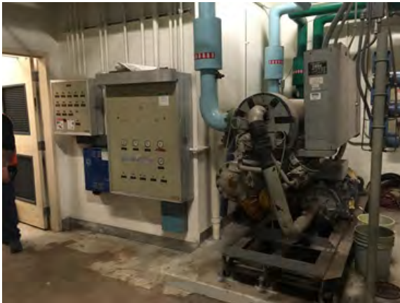
Fig. M-3 – Small Abandoned Chiller
