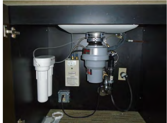
Fig. P-19 – Under sink equipment – water heater, garbage disposal, and filtered water.
