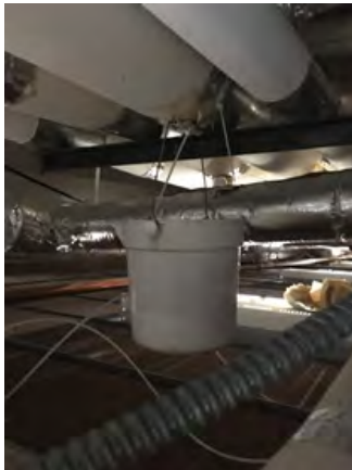
Fig. M-2 Bucket Below Heating Water Piping
