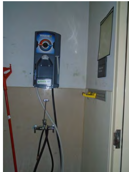
Fig. P-21 – Typical mop sink soap dispenser
