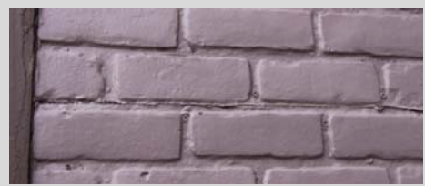
This detail of Building B shows a painted brick façade, with closer review revealing the screws that fasten the plastic bricks to the wood structure
